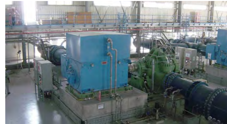
Figure 1 Water Transmission Pump
