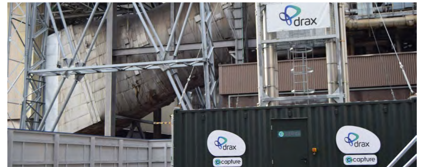
C-Capture's BECCS pilot plant operating at Drax Power Station, N. Yorkshire, UK
