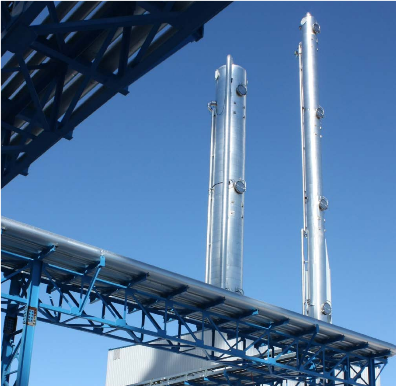
Figure 4 – Saipem CO 2 Solutions’ Pilot Plant in Québec, Canada (Source: Saipem)
