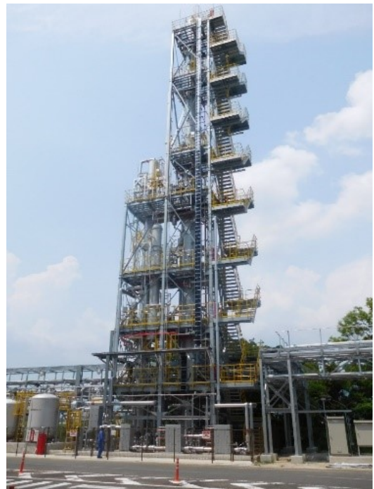
Figure 8: Carbon capture plant at Saga City WtE plant, Japan (image supplied)
