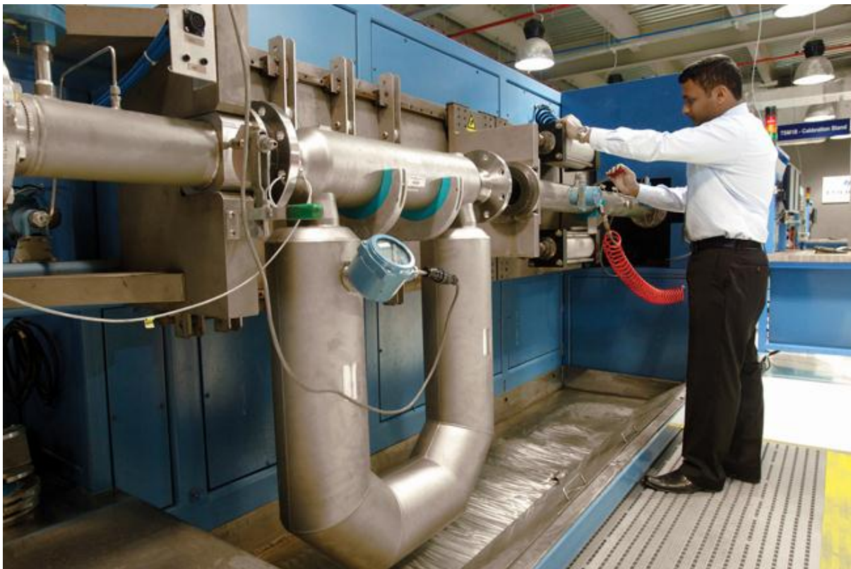
Figure 3.9 Coriolis Flow Meter (probably a 6 inch meter, available up to 12 inch, DN300)
